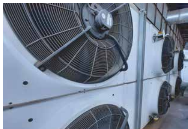
Using generator radiator instead of cooling tower
