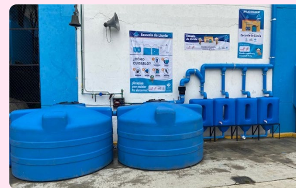
Image: Rain water harvesting in Mexico City
